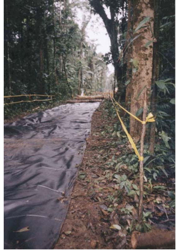
Fig. 6 – Geotextile and riprap installed to support the weight of the pipe carriers and protect tree roots in the thin rainforest soils.
