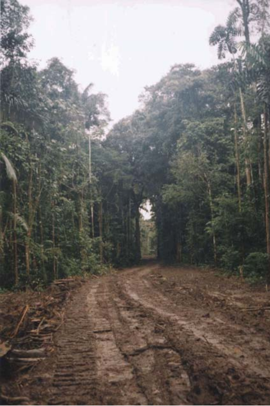
Fig. 5 – The 15 meter wide ROW of the pipeline, which narrows to seven meters to form a canopy bridge.
